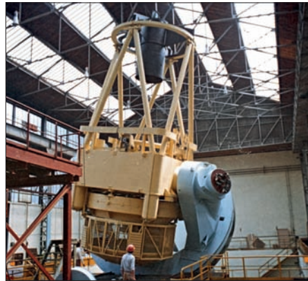
Main structure of the ESO 3.6 m telescope during assembly in France before shipping to La Silla, in Chile.
